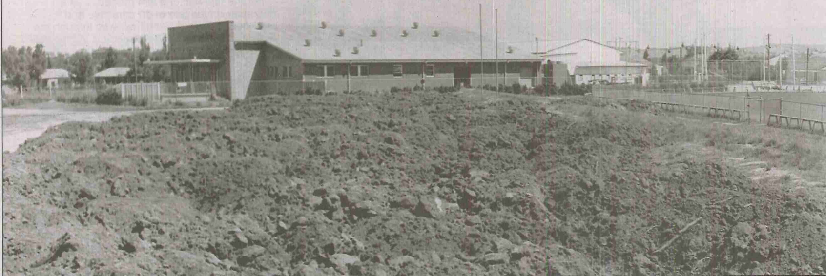
The construction of "The Hill" on the eastern side of Eric Weissel Oval, taken before 1964. From the left can be seen the new Wagga Leagues Club building, the original clubhouse (now the tennis clubhouse), the newly constructed tennis courts and Eric Weissel Oval (from the Tom Lennon Collection, RW1574/852).
