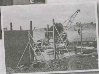
BELOW: This image shows the RVN 2 station under construction in September 1963. Two things of note are the empty paddocks behind the houses in Lake Albert Road and the workman riding the crane hook.
