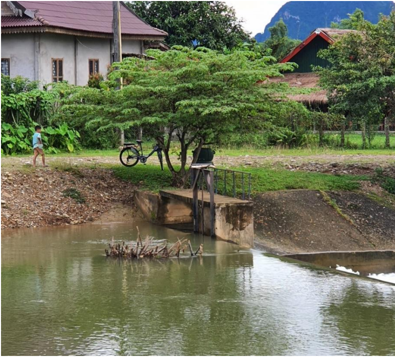
Photo 4. Gate adjacent to fishway which community members are concerned about, Nam Pok, Laos
