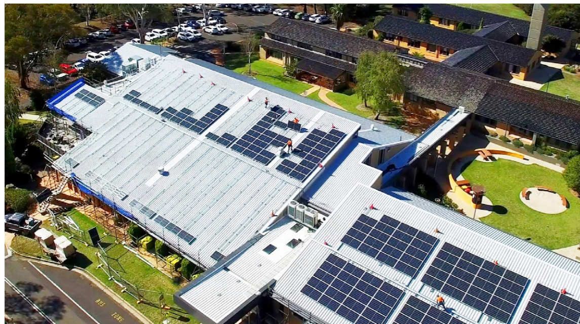
Solar installation at Orange Campus.
