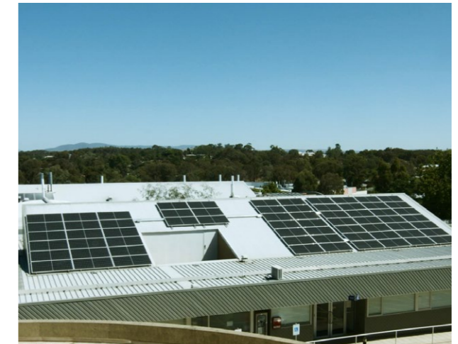
Solar photovoltaic installation as part of stage 2 in Albury-Wodonga
