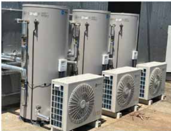
Reclaim hot water heat pump manifold
