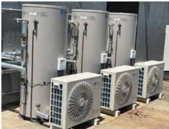
Reclaim hot water heat pump manifold
