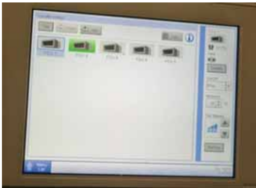
McDonoughs – Uncommissioned BMS
