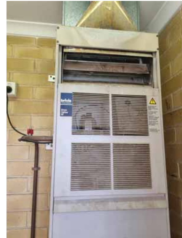
Windradyne – Ducted gas heating system
