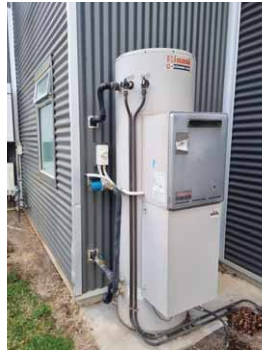
Macquarie Village - Gas hot water system
