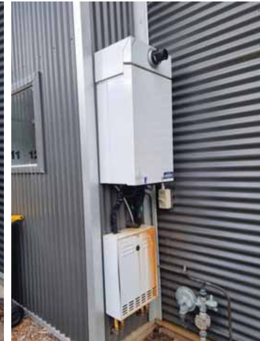
Macquarie Village - Gas hydronic heating system
